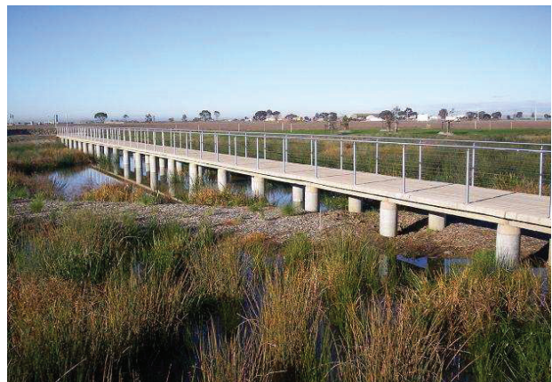
PermaTrak boardwalk over wetlands - Australia
